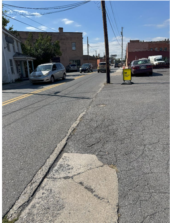
Figure 6. Deficiencies in sidewalk conditions along portions of Winchester Avenue, as shown here near 205 Winchester Avenue.
