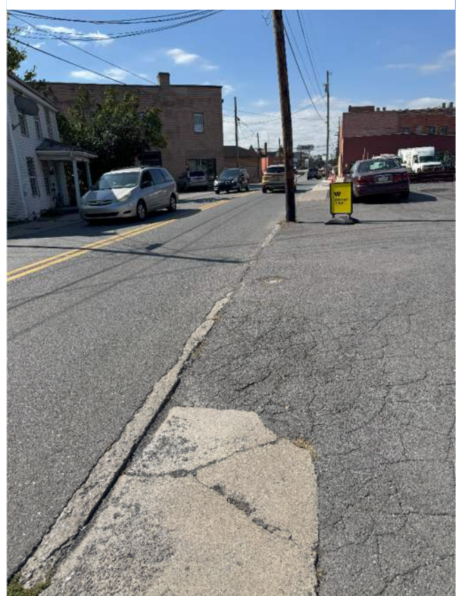
Figure 6. Deficiencies in sidewalk conditions along portions of Winchester Avenue, as shown here near 205 Winchester Avenue.
