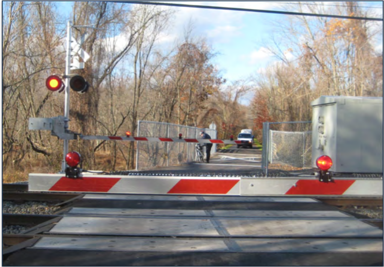
Photo of an Ideal At-Grade Pathway Crossing with enhanced Safety Features and Warning System
