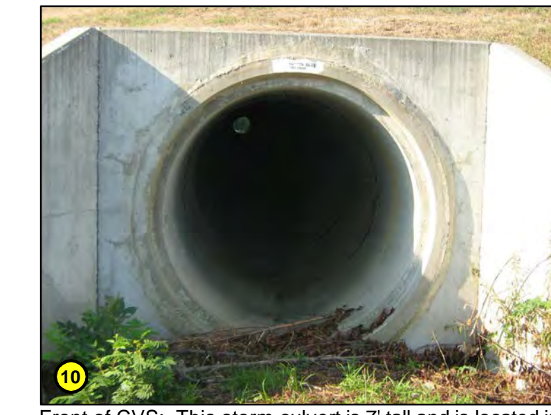
Front of CVS: This storm culvert is 7' tall and is located in the vicinity of the proposed trails southern terminus. Separation between the pedestrian route and the steep slopes & culverts in this area is necessary.
